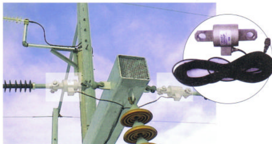
Load cell installed at deadend structure
