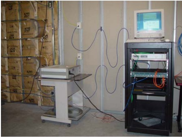
Figure 2: Haefley Generator and Cisco Switch
