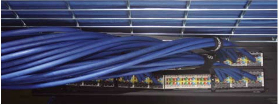
Pictured are two Ortronics' stacked overhead patch panels, offering a flexible solution and reducing valuable space within the racks and cabinets.
