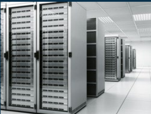
Telecom & Data (covering data transmission, telecom networks, hyperscale data centers, LAN)
